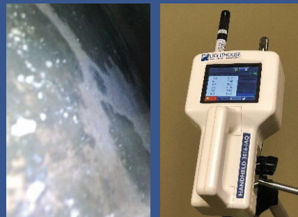
Left: Mold growth found within wall cavity by inspection camera Right: PM10 & PM2.5 Particulate Testing
